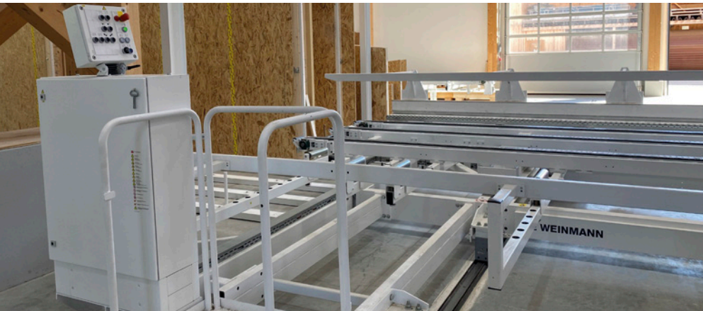
Traveling control panel
